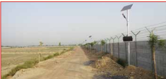
■ Solar street lights spread in the entire campus
